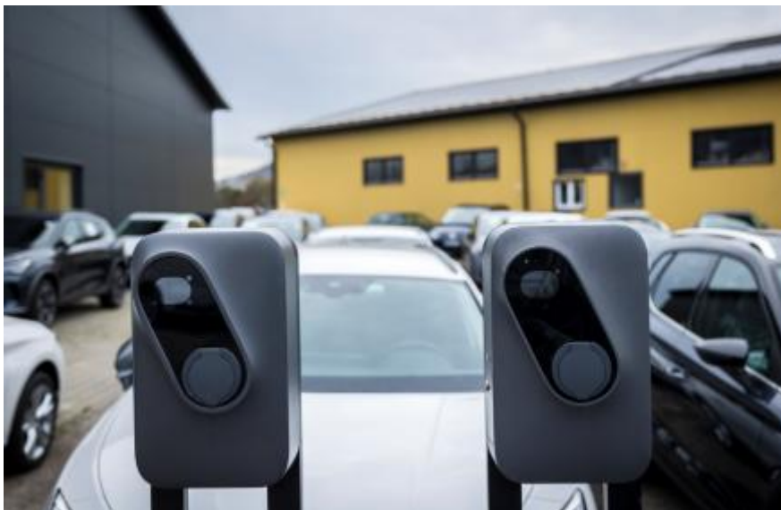
Figure 7 EMS (Emobility Solutions) charging station
