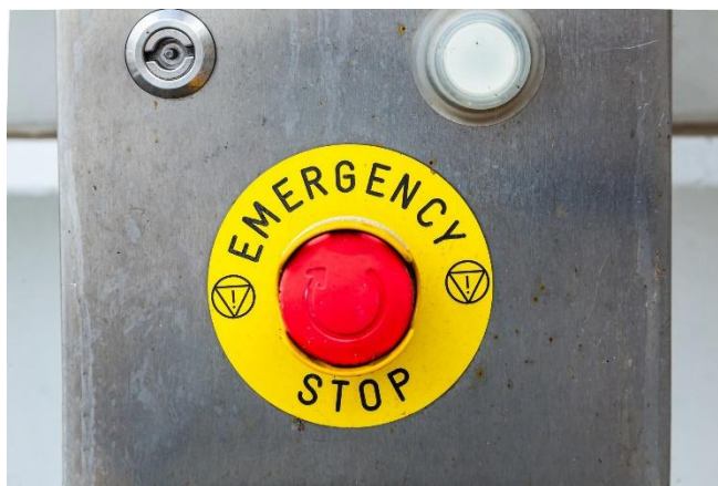
Figure 23 Emergency disconnect button on the charger
