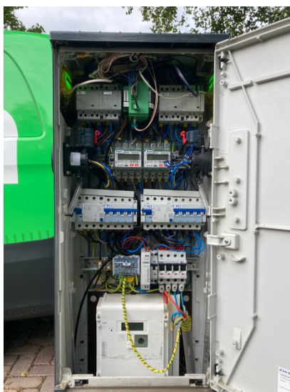
Figure 25: Refurbishing the V2G chargers of We Drive Solar to meet the ISO15118-20 requirements
