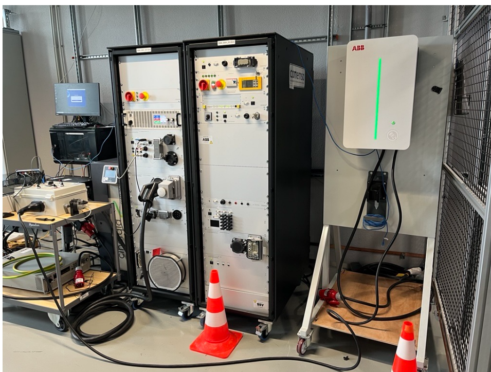
Figure 13: Test setup of V2G charger in the ABB lab environment
